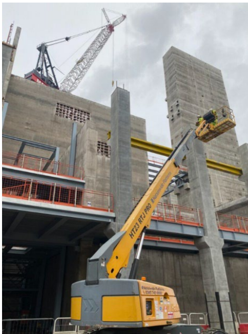
Figure 3: Support columns ready for the administration building floor. The yellow rails form the crane system which will allow a 'grab' to move ash waste from the boilers into trucks ready to be recycled
