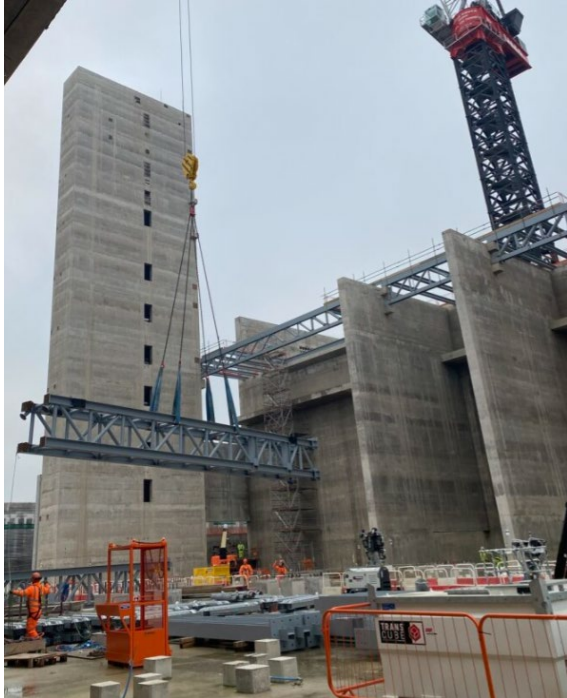
Figure 1: In scope mechanical works include steel columns for flue gas treatment equipment and roof support
