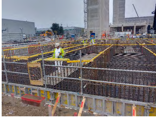
Figure 1: Substation concrete foundation slab for substation, one of the last deep pours.
