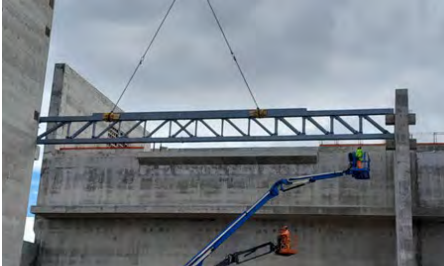
Figure 5: Installation of horizontal steel members and edge protection in preparation for deck installation
