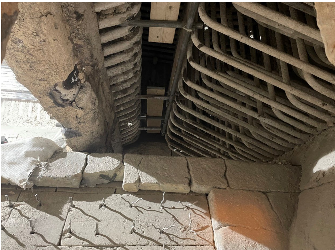
Figure 2: Steam tubes inside a boiler. Fixing some tube leaks requires Oxy-acetylene cutting and removal of healthy pipes to access the fault.
