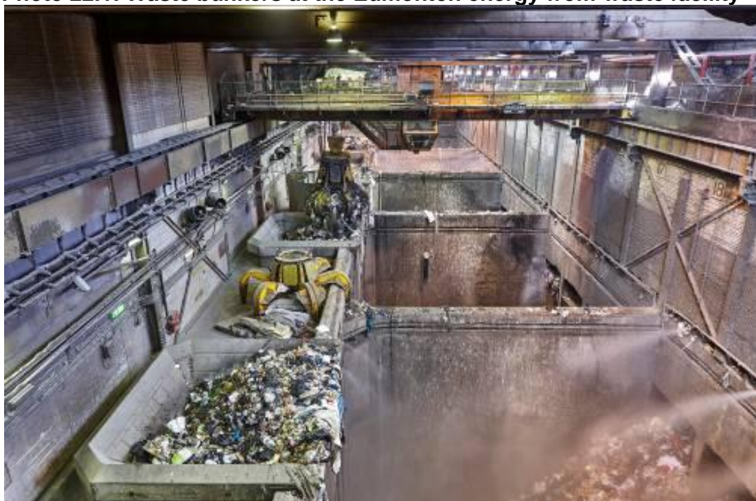
Photo 22.1: Waste bunkers at the Edmonton energy-from-waste facility
