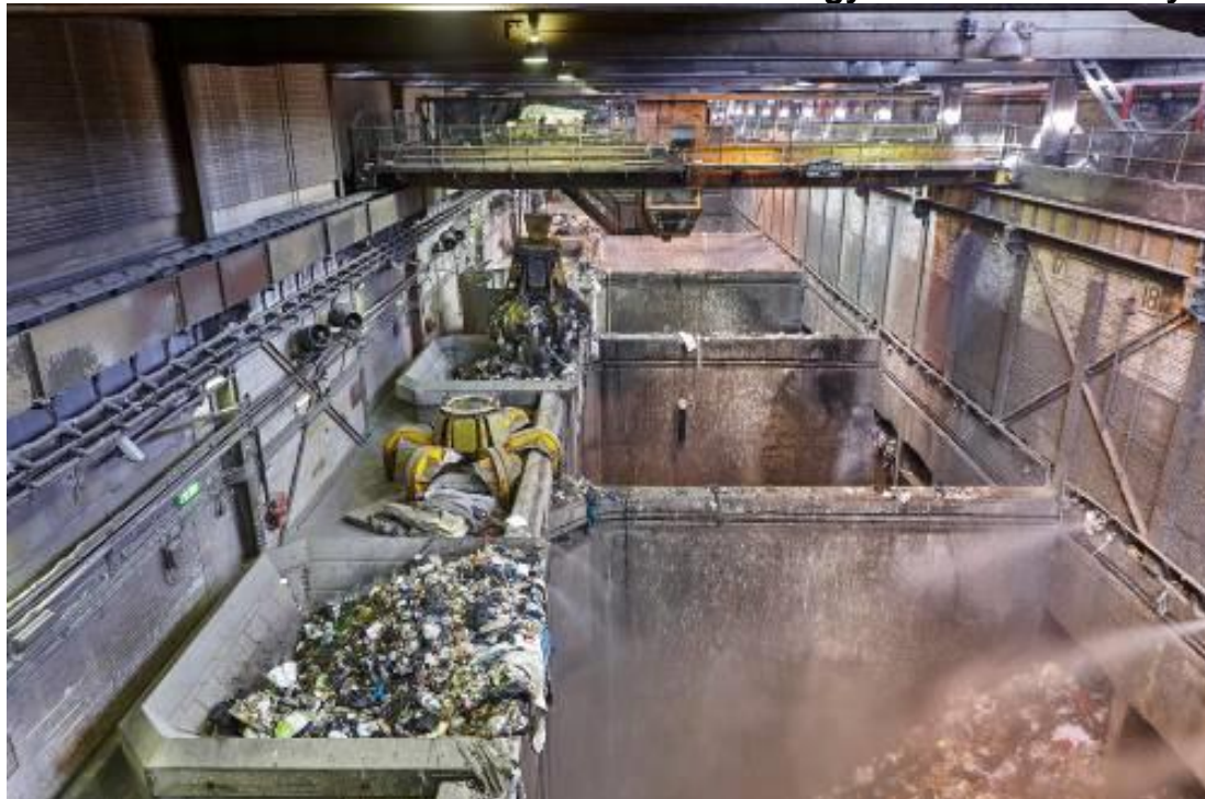
Photo 22.1: Waste bunkers at the Edmonton energy-from-waste facility
